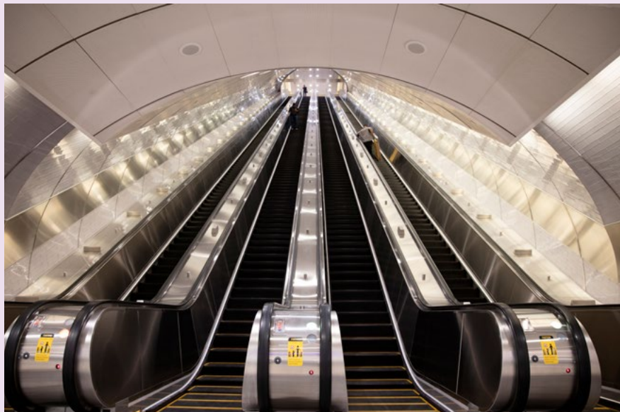
Escalators in the new Grand Central Madison terminal
